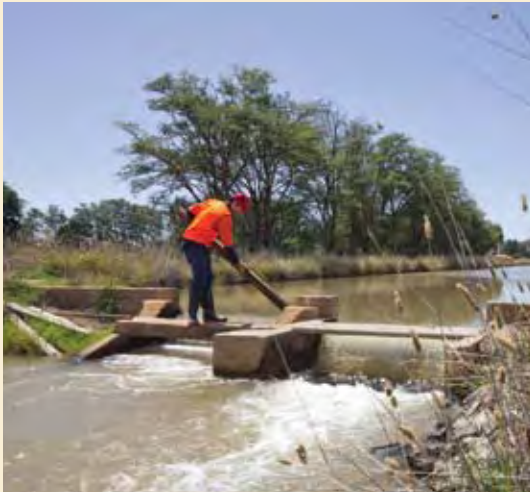
Manual regulating control structures
