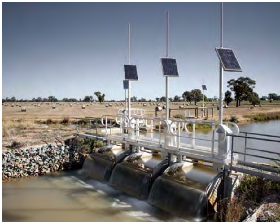
FIGURE 4 FLUMEGATES FEATURING INTEGRATED ACTUATION, WATER LEVEL AND FLOW MEASUREMENT
