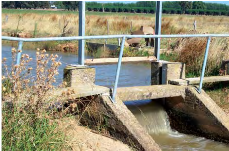
FIGURE 2 AGEING IRRIGATION INFRASTRUCTURE
