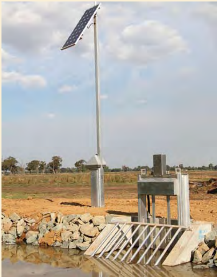
Automated integrated metering (Rubicon SlipMeter™)
