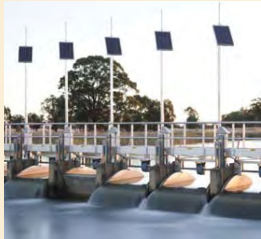
Automated control structure
